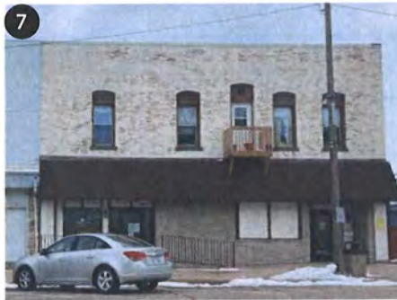
7 140 E Oak St Major Improvements Needed
