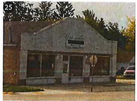
207 West St Major Improvements Needed
