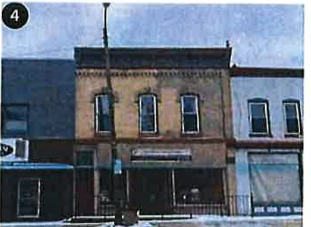
120 E Oak St Major Improvements Needed
