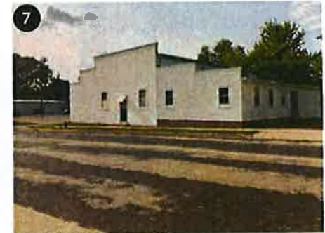
224 N Depot St Major Improvements Needed
