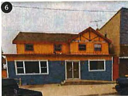
6 130 E Oak St Major Improvements Needed
