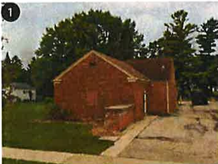
228 E Center St Major Improvements Needed
