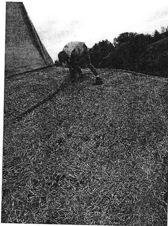
Photo 4: Securing erosion control fabric along northwest corner of gypsoil building. Date of photo May 2021.
