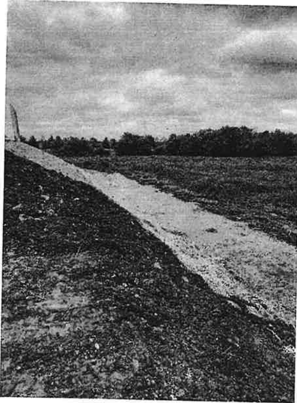
Photo 3: Erosion control fabric being placed over newly seeded areas. Date of photo May 2021.
