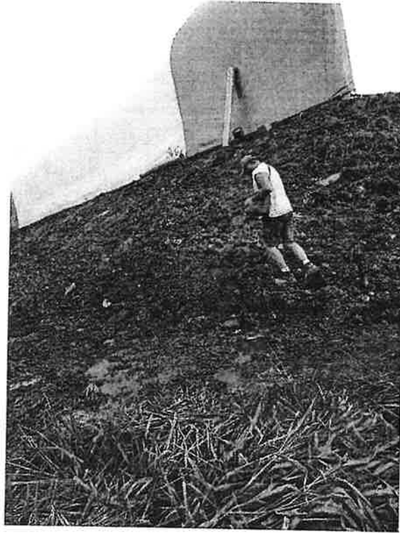
Photo 1: Looking south at gypsum building showing excavated side-slope. Date of photo May 2021.
