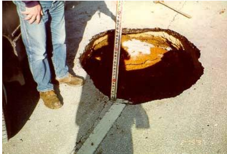
Sinkhole in Monroe County, WI
