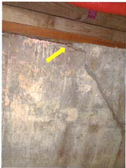
Falling below sill plate
