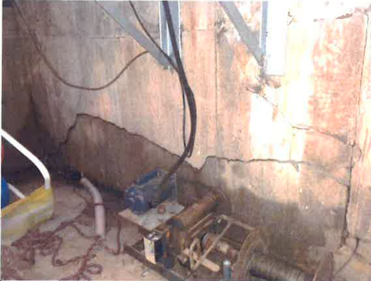
Foundation failure East wall
