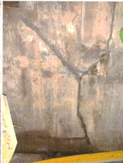
Foundation failure South wall
