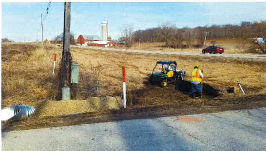
Installing new culverts and erosion control measures near the Schwarze Road crossing.
