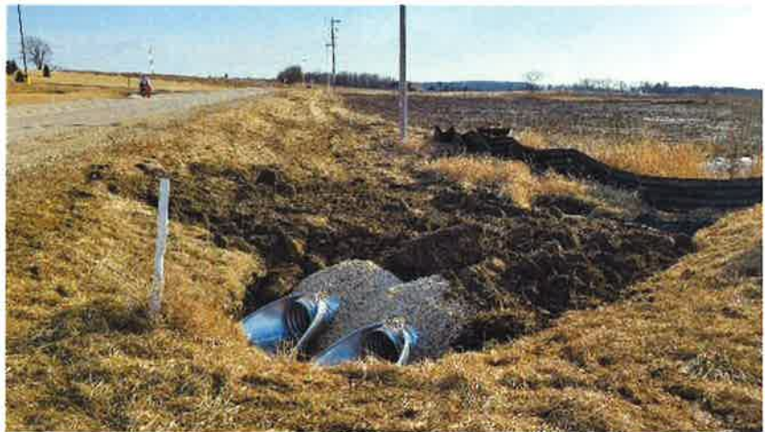
Installing silt fence and new drainage culverts along STH 28 for the new trail.
